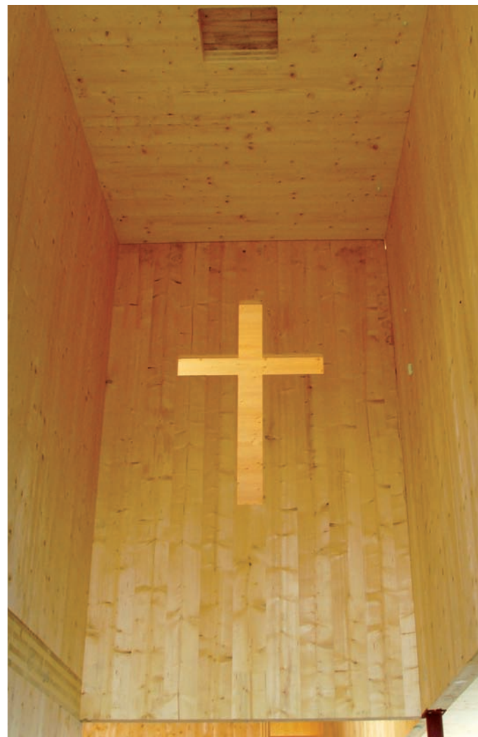
Timber panels were treated with intumescent varnish and lined in some places with MDF.
