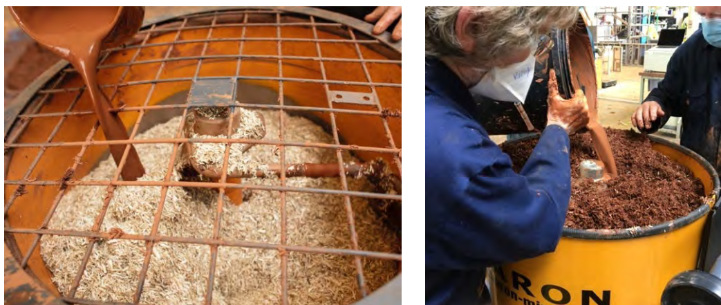
Figure 10. Mixing of the clay slip and hemp shiv fibres off site using a baron mixer. Photos: Plymouth University.
