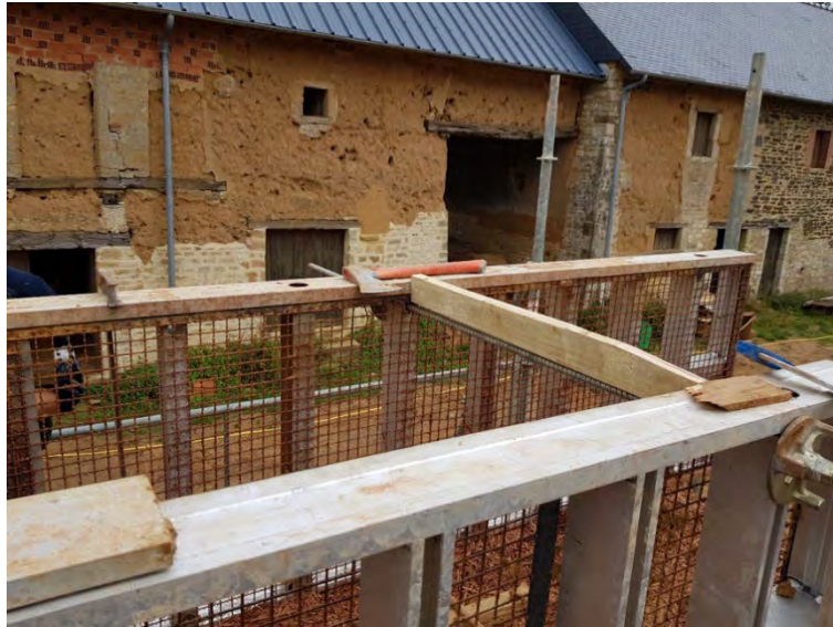
Figure 24. Photo showing spacing of formwork using wooden spacing block. Photo: François Streiff.
