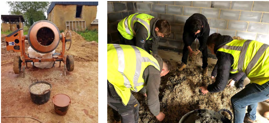
Figure 9. Mixing of light earth mix on site using a cement mixer (left) and by hand (right). Photos: François Streiff (left) & Anthony Hudson (right).
