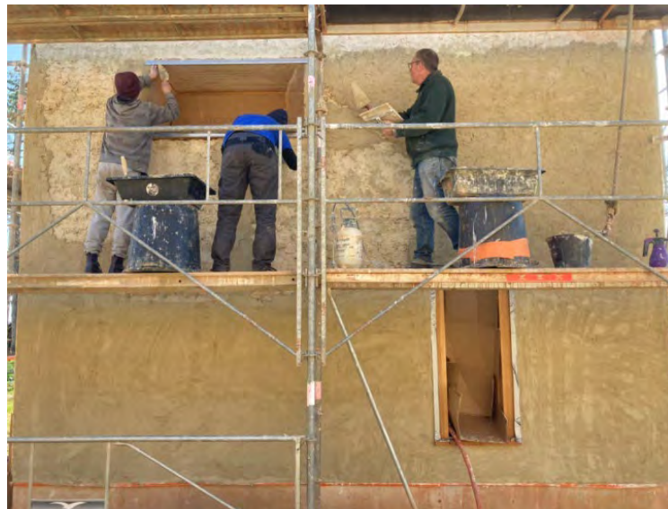
Figure 44. Example of lime render being applied to a CobBauge wall. Photo: Raphaël Rattier.
