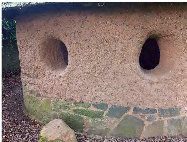
>>> Photo 3. Rammed earth walls in a shelter on a recreation ground at Letham, Angus. Constructed using glacial till derived from local Devonian bedrock and designed by Arc Architects Ltd. Photo TD Holt-Wilson.
