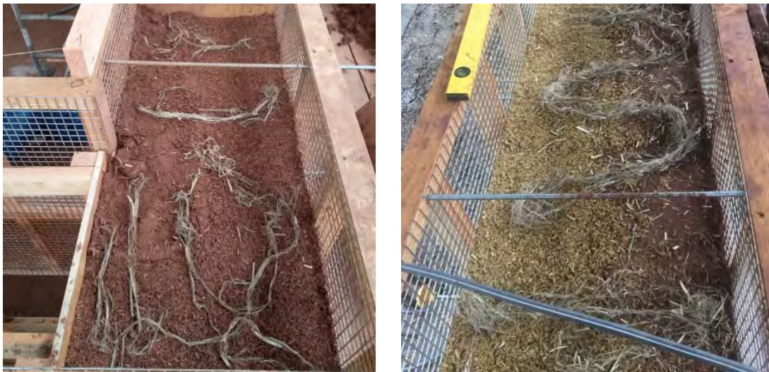
Figure 29. Hemp straw placed, after each sub lift, perpendicular to the run of the CobBauge wall. Photos: Jim Carfrae.
