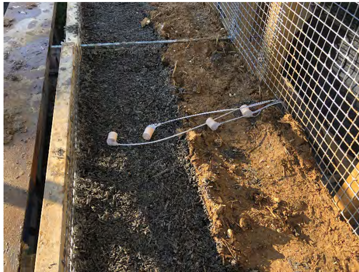
Figure 37. Ramin Sensors laid in place, ready to be embedded into the final CobBauge lift. Source: Anthony Hudson.
