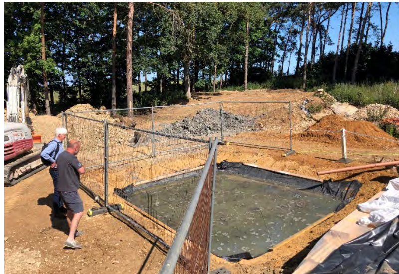
Figure 5. The thermal mix subsoil soaking in a watertight pit. Photo: Tom Boen.
