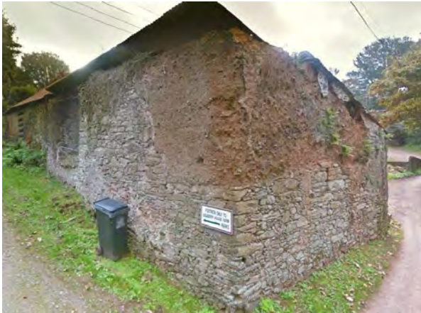
Photo 8. A cob wall with stone footings at Bolberry, Devon, made from local head deposits derived from Devonian bedrock. The material is exposed to rainwash and freeze-thaw erosion where a sheltering roof is missing. Photo courtesy Google StreetView Oct. 2016 © Google 2022.
