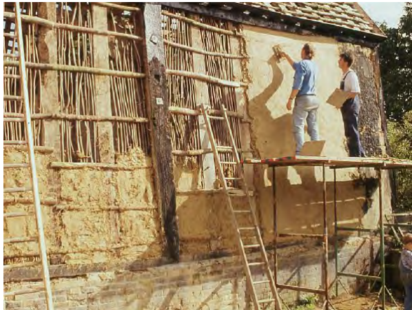
>>> Photo 1. Restoring a 16 th century barn at Dairy Farm, Newton Flotman, Norfolk, 1992, with wattle and daub technique using Lowestoft Till puddled with chopped straw. Photo TD Holt-Wilson.
