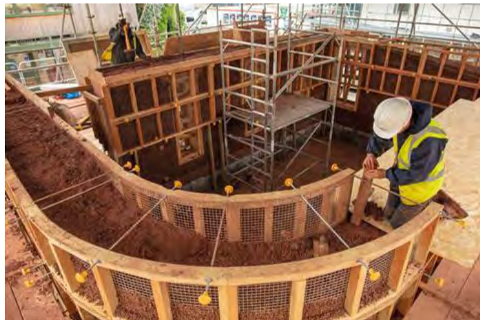
Figure 42. Scaffolding on the inner and outer sides of the CobBauge wall as it rises.
