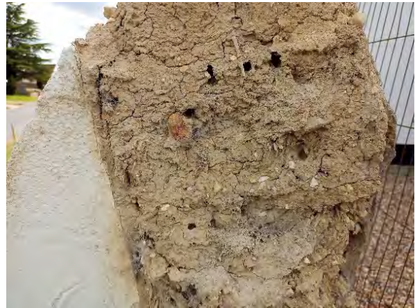
>>> Photo 2. A damaged farm yard wall at Finningham, Suffolk, showing crudely layered, cob construction, probably 18 th or early 19 th century. It is made of Lowestoft Till puddled with straw, set on brick footings and is faced with tar-painted plaster. Photo TD Holt-Wilson.
