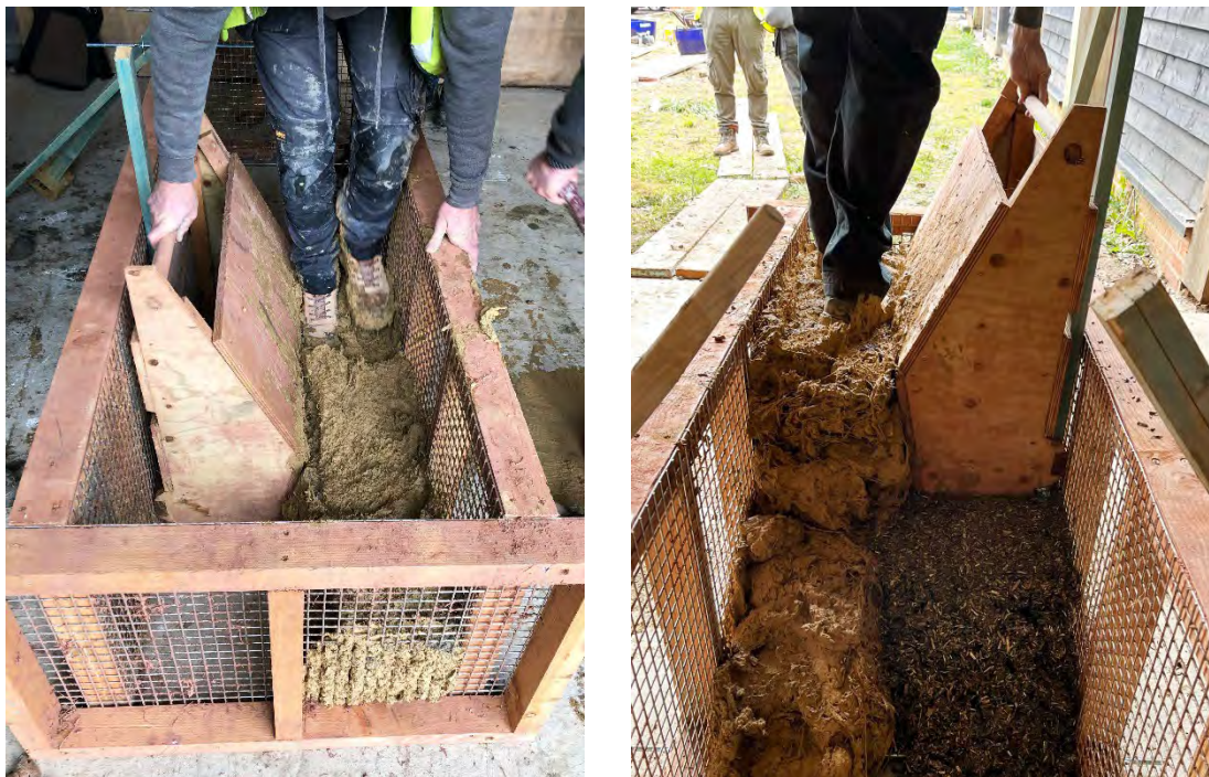
Figure 28. Placement tool and stamping compression technique for structural layer. Photos: Tom Booen.
